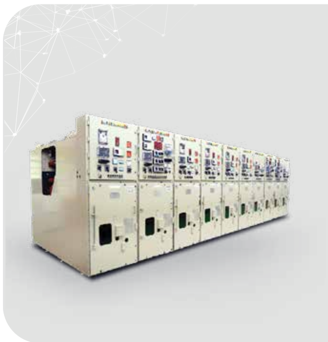
CG 3.3kV to 33kV Indoor VCB
