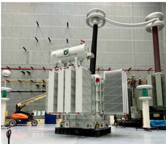
CG's 1-Phase Reactor, Mandideep Testing Lab, Madhya Pradesh, India
