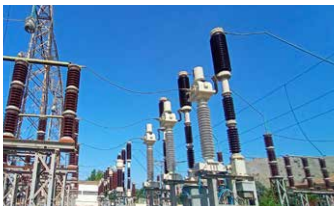
CG's 170kV Polymeric Current Transformers supplied for Caserta Substation, Marzanello, Italy
