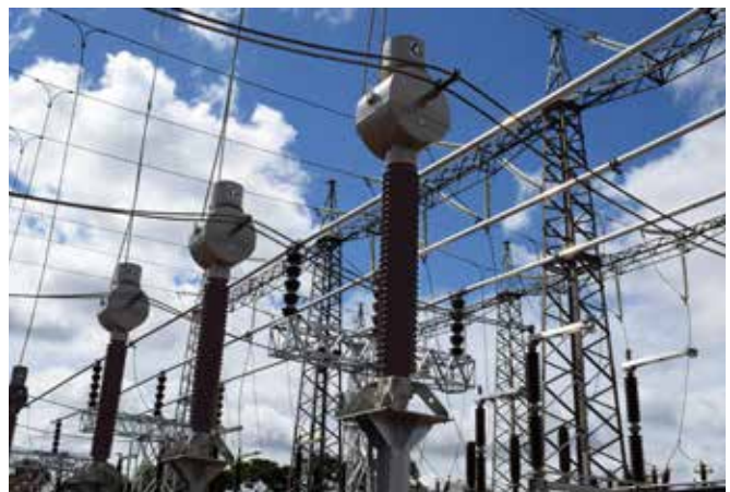
CG's 245kV Current Transformers In ANDE ACARAY Substation, Paraguay
