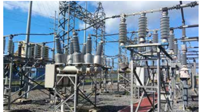
CG's 72.5kV Dead Tank Braker at Union Substation, Trinidad & Tobago, West Indies
