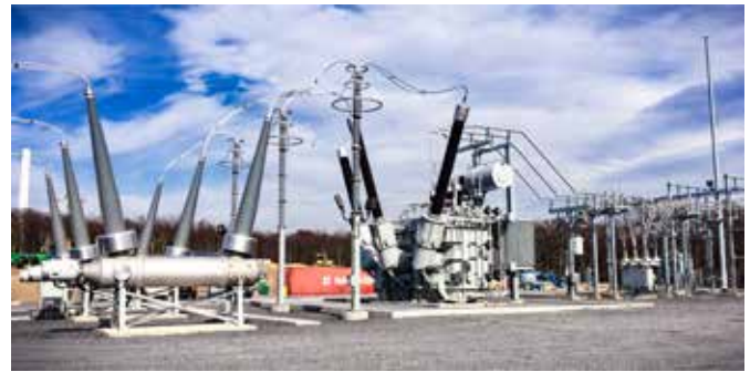
CG's 143MVA 500kV/34.5kV/13.9kV Power Transformer supplied for Enbridge - New Creek Wind Farm, West Virginia, USA
