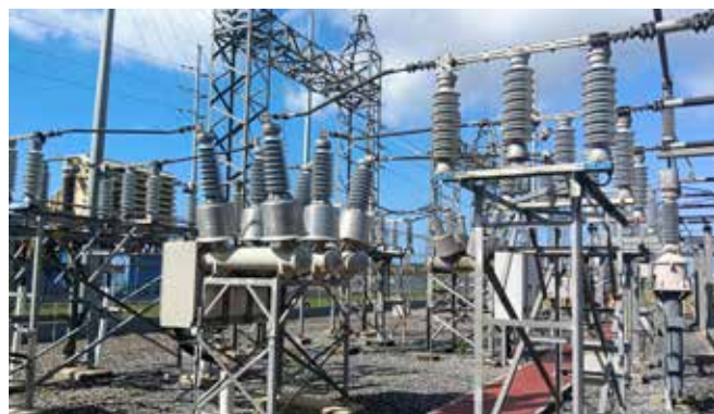
CG's 72.5kV Dead Tank Braker at Union Substation, Trinidad & Tobago, West Indies
