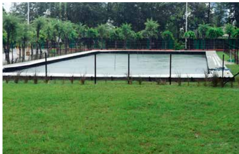
Rainwater Recharge system at LT Motors Unit-1 Facility, Ahmednagar
