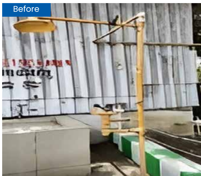
The eye-wash is used when some irritants enter the eye. It was stationed at a single place.
